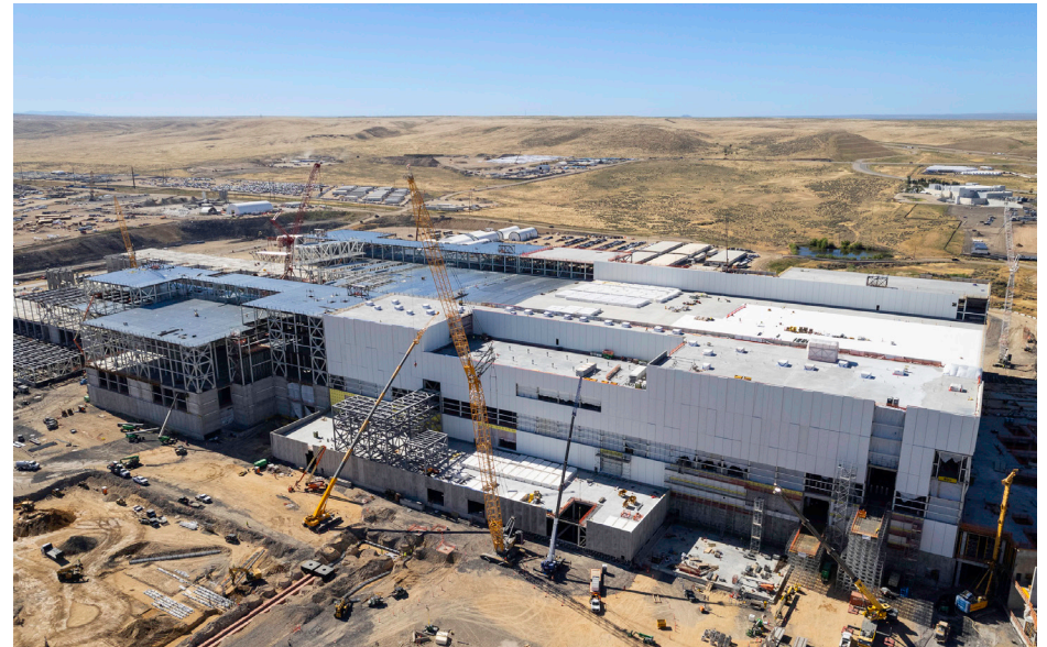
Construction on Micron's new semiconductor fabrication facilities in Boise was progressing in 2025 and had already hit key milestones. Image credit: Micron.
