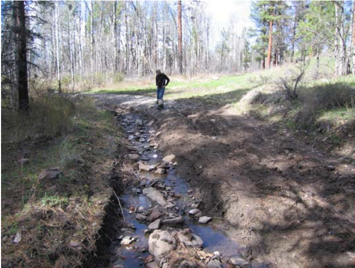
Photo 4: A stream channel that was ‘captured’ by a road creating severe erosion. A culvert will be installed to reroute the stream and the road surface will be leveled and rocked in October 2008.
