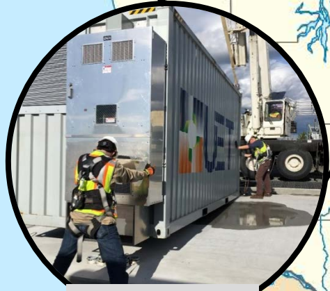
MESA 2 2MW/6.4MWhr $4.4M
